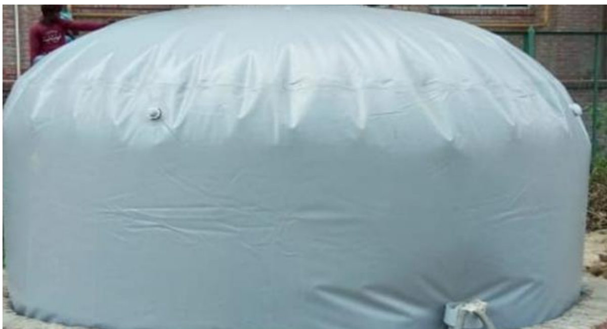
Fig.14.1. Biogas Plant near Block 7 (Sharda University)
