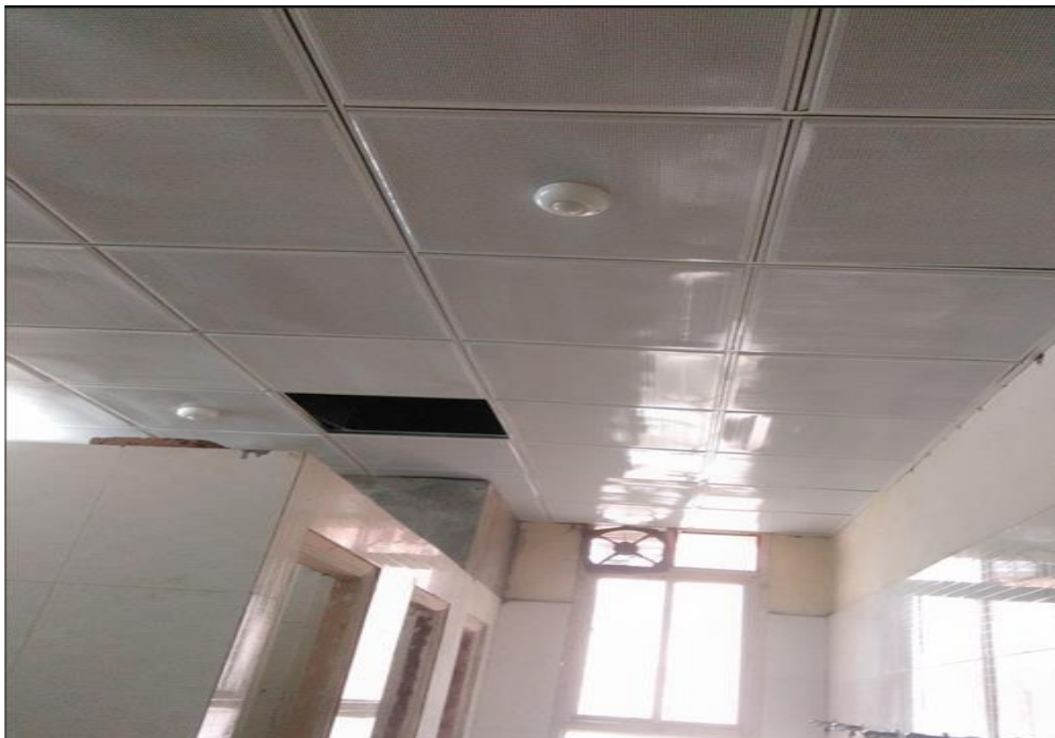
Fig.5. Sensor Lights in washroom
