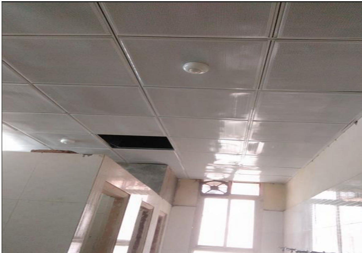
Fig.5. Sensor Lights in washroom
