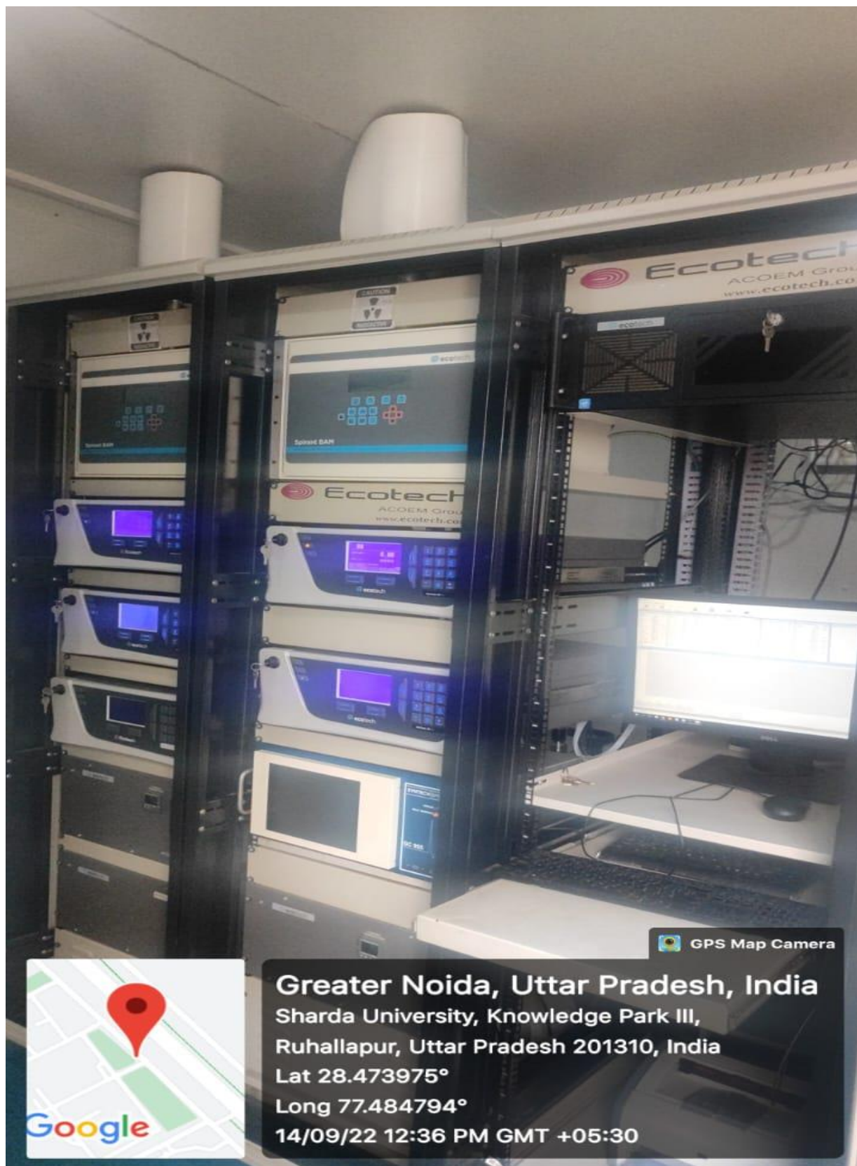
Fig.9. AQI room to monitor air quality
